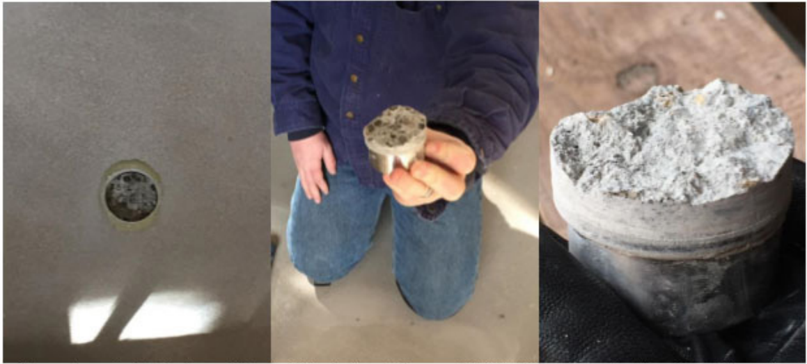
Fig. 3 – Concrete substrate being pull tested failed prior to Tremco PUMA Primer, showing the primer's tenacious bond.
